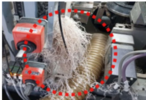
Insufficient Dust Collection
