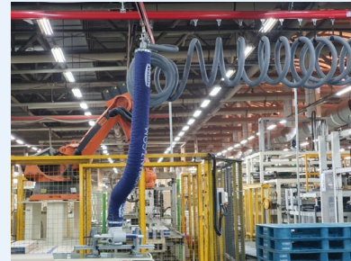
▲ Industrial Robot / Flexible Lift
